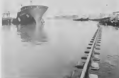
From this angle the floats alongside the Aquafence boom create an effect of a huge zipper. The boom runs parallel to the shoreline beyond Finger Pier # 3, from where it will be further extended to the Tugboat Dock seen at a distance.
